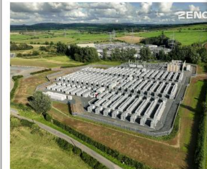
The 302 MW/500 MWh Kilmacknock South BESS represents a step up in the volume of inertial UK batteries are providing to the grid.
